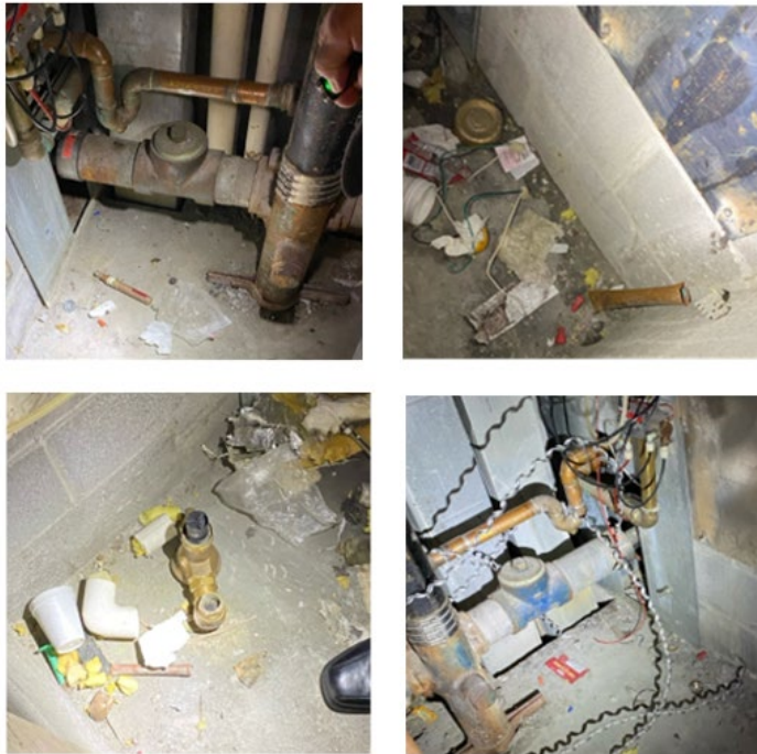
Unsecured pipe chases in the Jail
