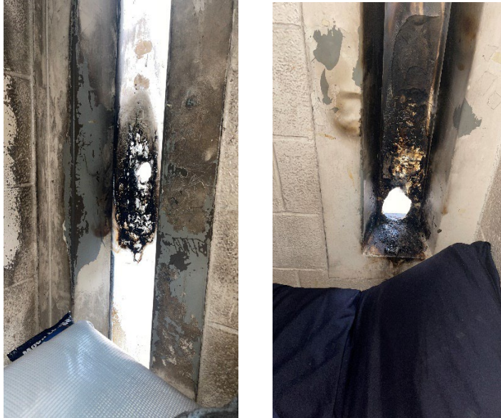
Burned holes in cell windows observed during DOJ October 2023 inspection
